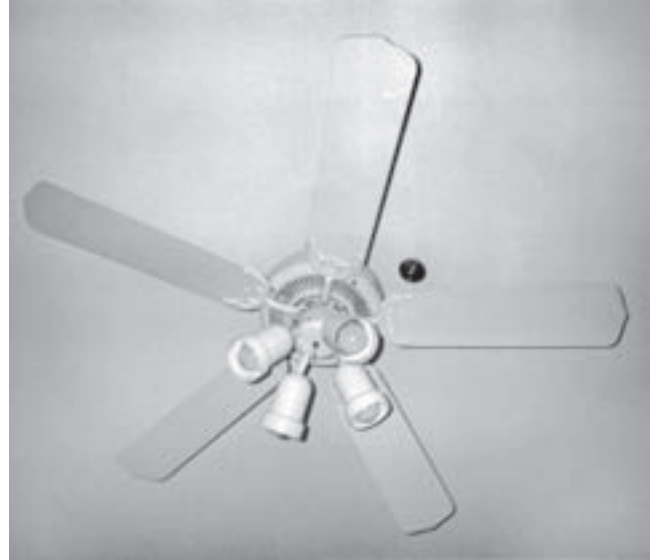
FIGURE 16.6.11 Residential Sprinkler Obstructed by Ceiling Fan
